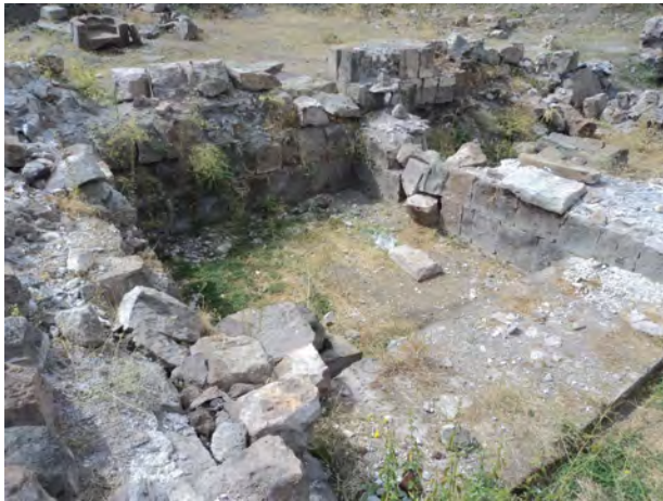
Figure 10. Medieval bath structure in Ahlat. The surrounding earthen fill, the exposure of the tops of the walls and the effects of the continental climate cause further structural losses in the building remains (photo by Şener, 2015).
