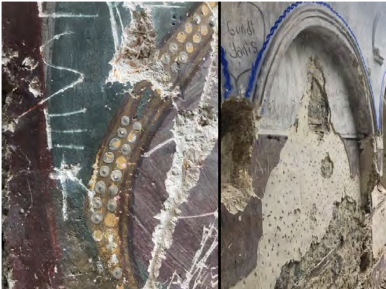
Figure 7. Vazelon Monastery (Trabzon, Türkiye), used from the Byzantine period until today. Right: Straw-added plaster material, which becomes visible thanks to spillage, and putty paints that have been embossed on the surface. Left: Notch marks on the wall painting showing the construction of new plaster over previous plaster (photos by Şener, 2022).
