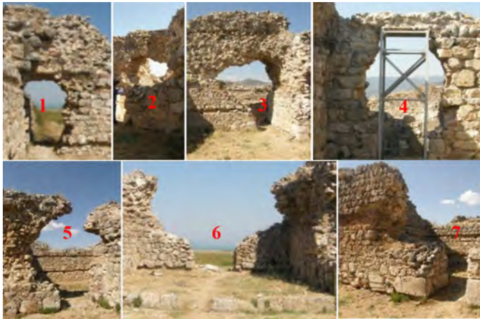
Figure 9. Seljuk period (13 th century) Kubadabad Great Palace Building (Beyşehir, Konya, Türkiye). Even from one's initial observations of the building, the stages of structural loss can be observed on the walls and around the door openings (photos by Şener, 2011).
