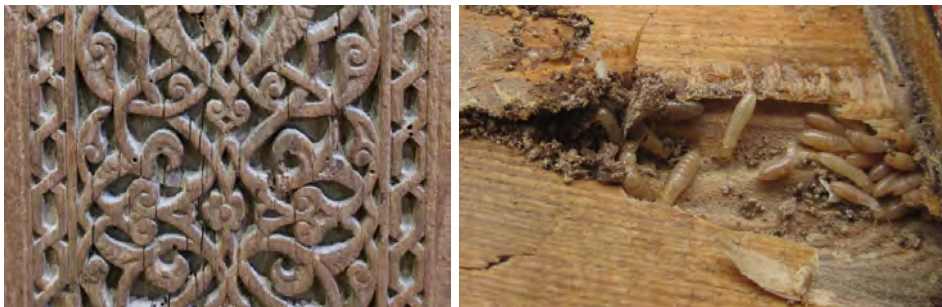
Figure 10. Longitudinal cracks and insect's exit holes on the decorated surface (left); termites in the window frame (right) (Photo. I. Özsait-Kocabaş).
