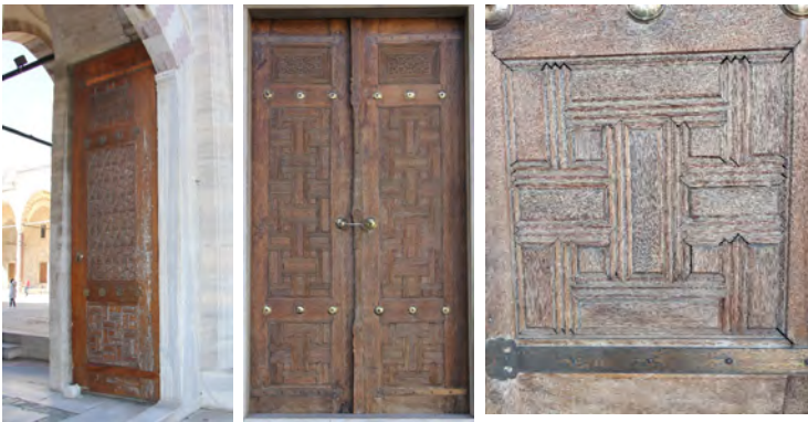
Figure 8. Loosening between wooden fragments, weathering, and discoloration on the mosque courtyard door wings (Photo. I. Özsaıt-Kocabaş).
