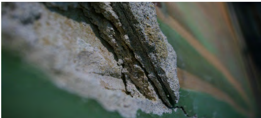
Figure 5. In situ delamination and detachment between preparatory layers due to shrinkage. Museo delle Arti e Tradizioni Popolari, EUR, Rome.
