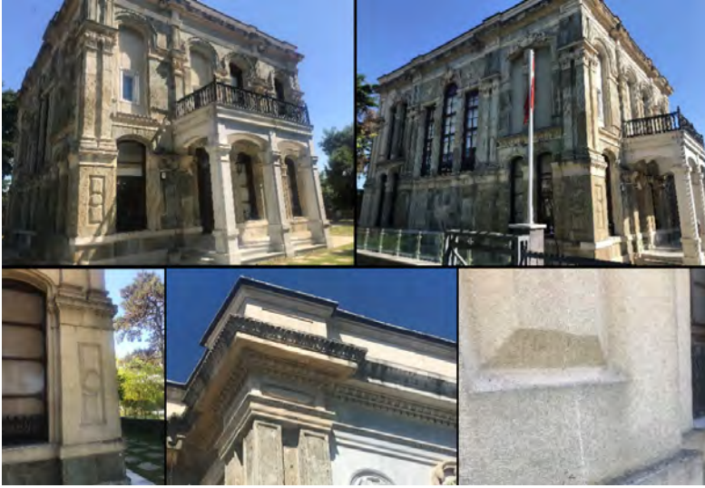
Figure 4. Reintegration applications using a type of limestone similar in color and texture during the 20 th -century repairs (bottom) in place of the tuff stone used in the original construction of the Abdülaziz Hunting Lodge (top) during the reign of Ottoman Sultan Abdulaziz (1861-1876; photos by Sener, 2022).
